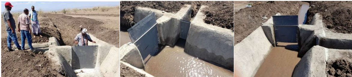
Fig 14: Canal control gates fixed in the division boxes
